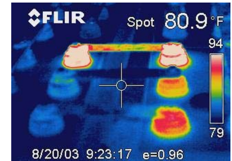
IR picture of a battery with a defective internal bridge.
